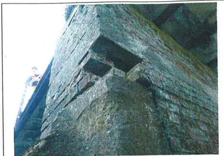
Photograph No. 3: Missing brickwork to the central pier
