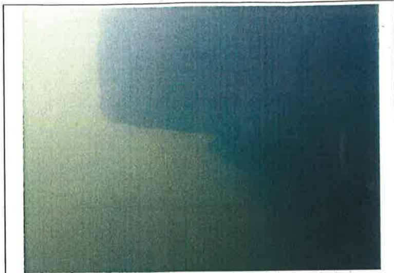
Photograph No. 1: Scour to the cutwater of the central pier
